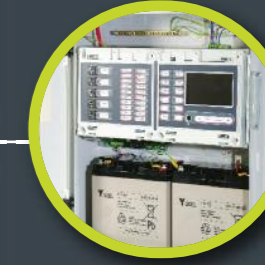
Up to 72 hours standby in standard cabinets
